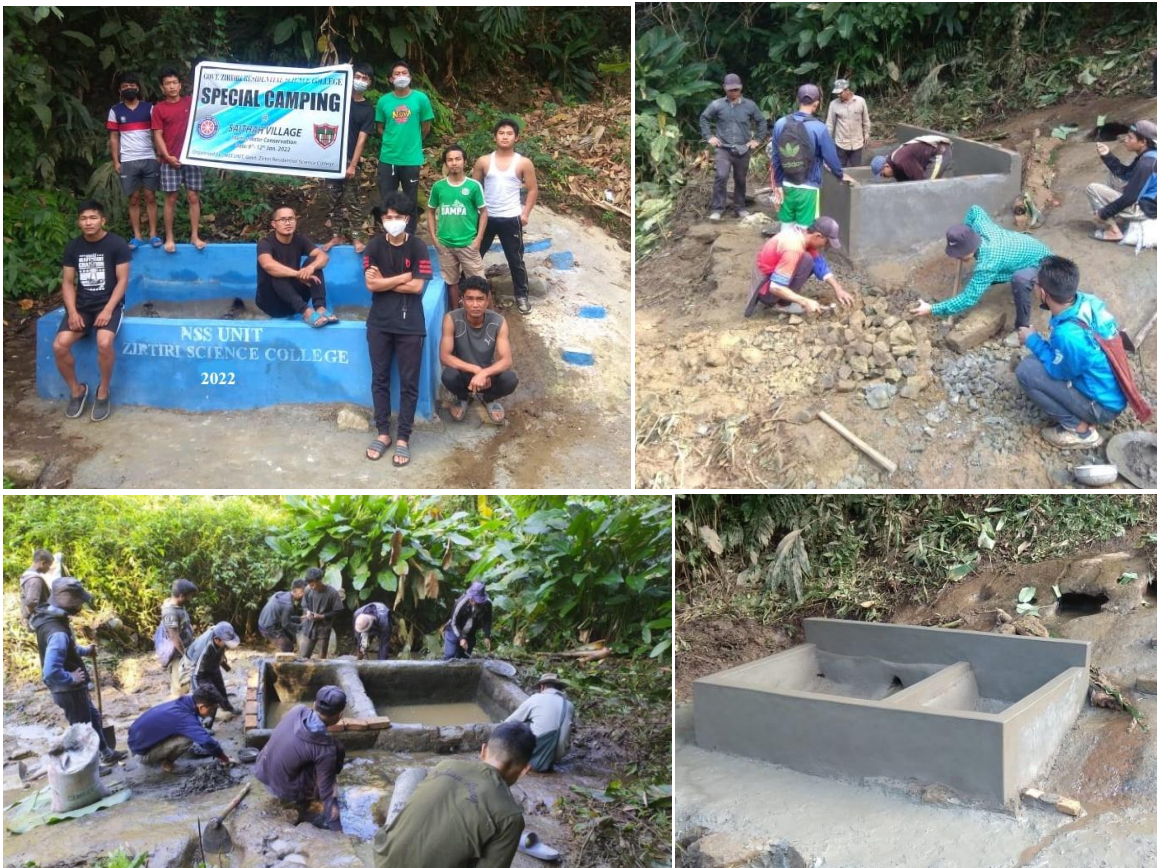
Special Camping at Saithah Quarry Veng (Construction of Water Reservoir) during 6 th – 12 th January, 2022
